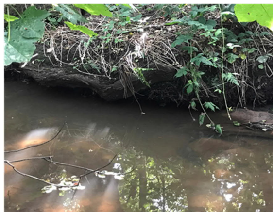
Plate 27: Watercourse 5a undercut bank
